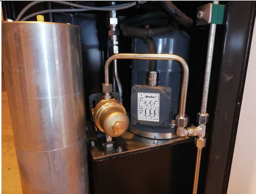
Picture 2 Example of hydraulic arrangement with new filter after modification
